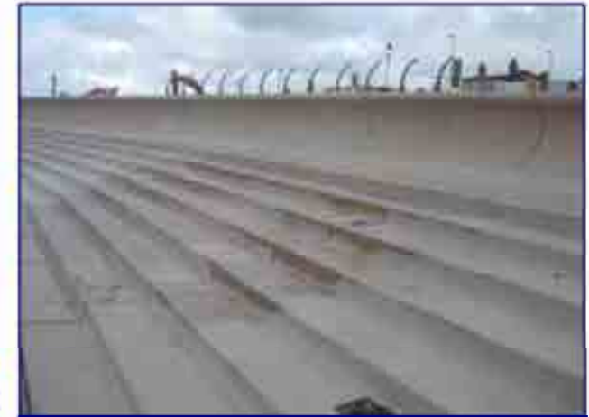
Example of what the new stepped revetment could look like, taken from Blackpool
